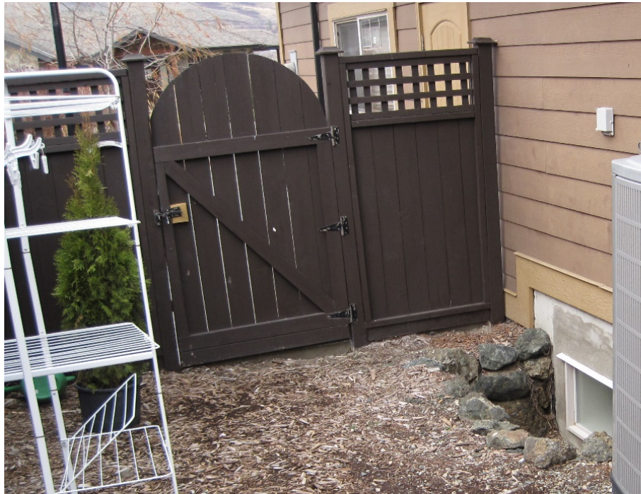
Figure 12 This wood fence bisects a bark mulch bed and connects to the house. Embers could ignite the bark mulch, leading to the fence catching on fire and posing a threat to the attached house. Note: this photo is not from Twin Lakes.
