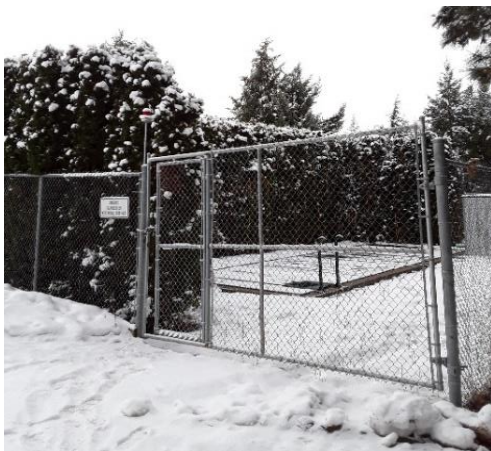
Figure 2: Westridge neighbourhood water pump and reservoir with highly flammable cedar hedging surrounding it (credit: M. Nederend, BA Blackwell & Associates Ltd)
